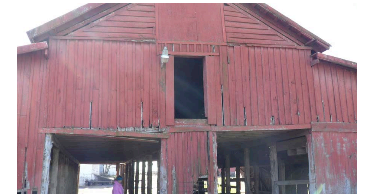
Figure 1. An aging barn originally built for housing cattle on the Lush Acres Farm at the Thornwell Home for Children. The barn has been designated for housing small ruminants (goats and sheep) or poultry (turkeys). Structural and cosmetic work is planned for the barn. Initial work has included cleaning out stall and storage areas in the barn. Repair work will involve structural improvements to the internal frame and external woodwork.
