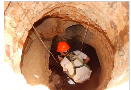
Dan Hitchcock, a faculty member for the Aiken Hydrological Evaluation project team, surveys stormwater drains in Aiken.
