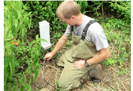
Graduate student Jeremy Pike installs a MoteStack at the Hunnicutt Creek stream restoration project site on campus.
